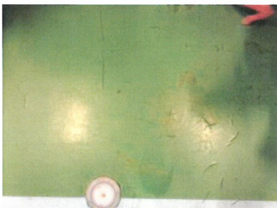
Revner i sportsgulv
